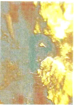
Actual photo taken by remote controlled camera showing grease buildup in sewer pipe interior.
